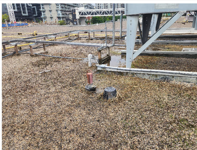
19 Description: Overview of large amounts of organic debris around the roof drain.
