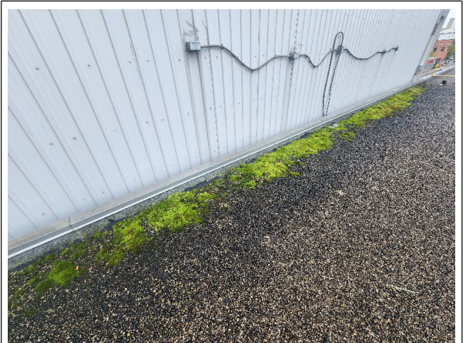
④ Description: An abundance of moss along the front of the building, indicating excess moisture sitting along the wall.
