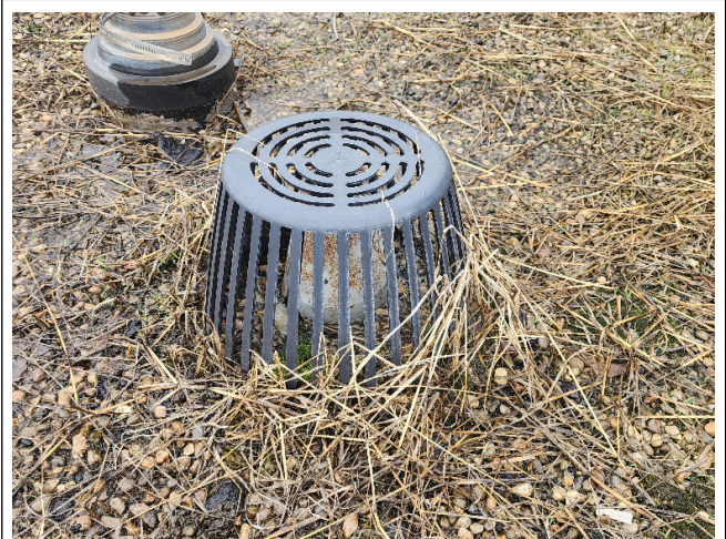
20 Description: Organic debris built up around the roof drain not allowing for proper drainage.
