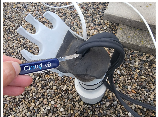
18 Description: Open sealant at a roof cone.
