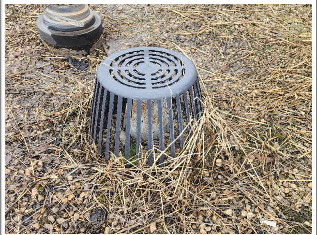
20 Description: Organic debris built up around the roof drain not allowing for proper drainage.
