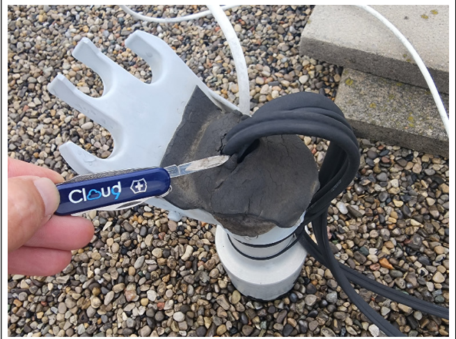
18 Description: Open sealant at a roof cone.
