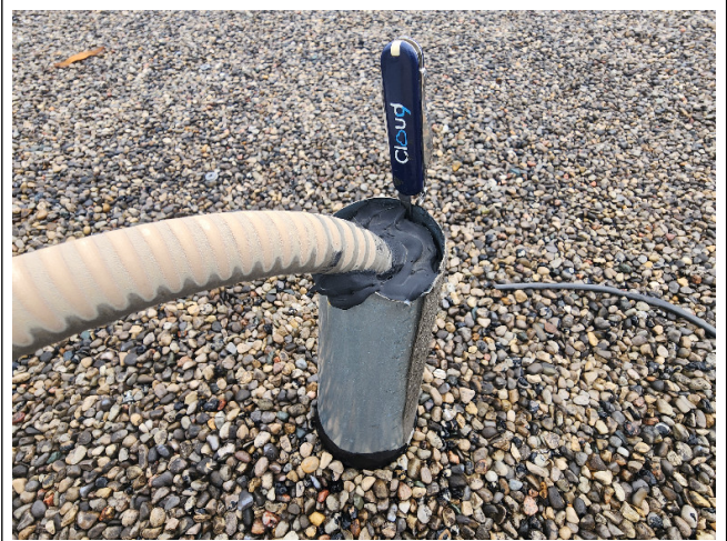
10 Description: Opening in the sealant of the cone.
