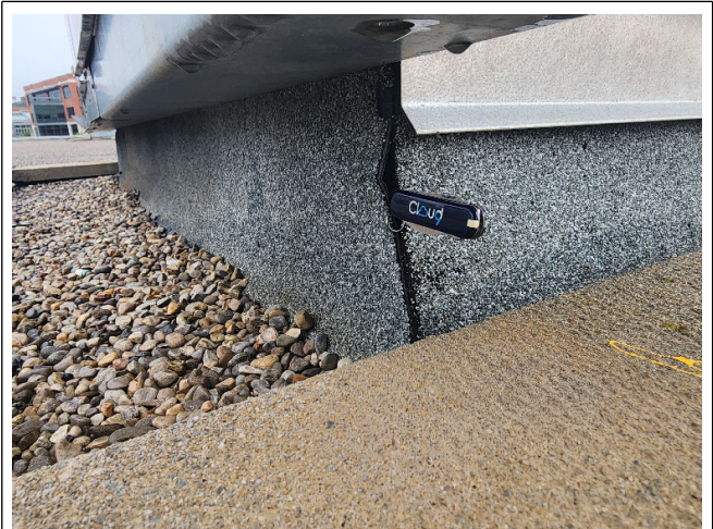
12 Description: Opening in the flashing under the HVAC unit allowing for moisture infiltration.
