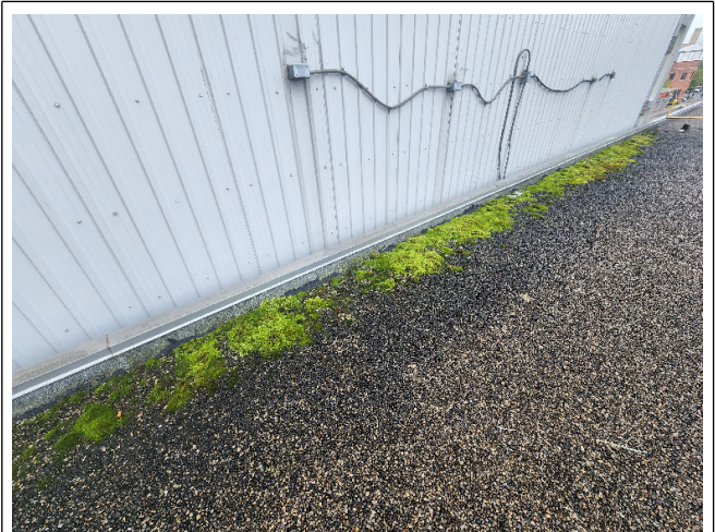
④ Description: An abundance of moss along the front of the building, indicating excess moisture sitting along the wall.
