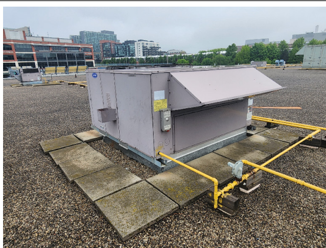
11 Description: Typical HVAC unit on this roof level.
