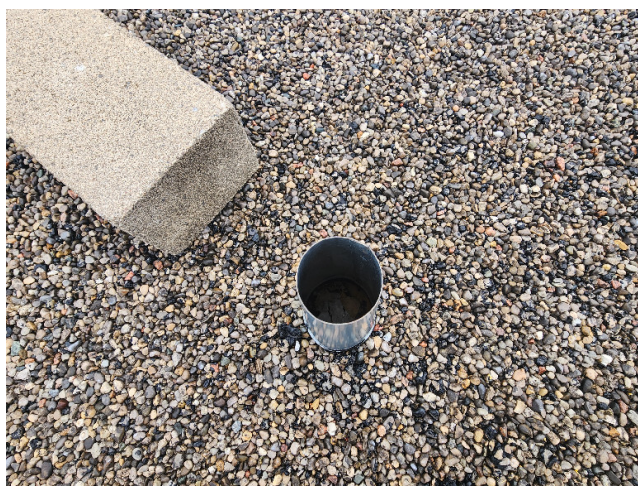
9 Description: Open roof cone will need to be covered to prevent water and debris to enter.
