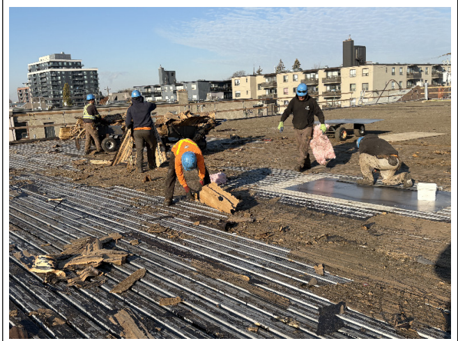
⑥ Description: The roofing crew removing the existing vapour retarder from the metal deck before starting the new roof build-up installation.
